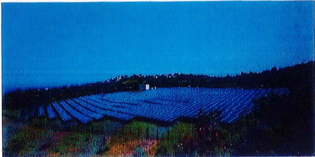
Figure 4 : Photos de structures fixes (source : SUNPOWER)
